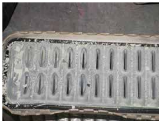
End tubes have become soft and distorted.
