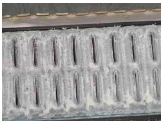
Header plate showing white deposits.
